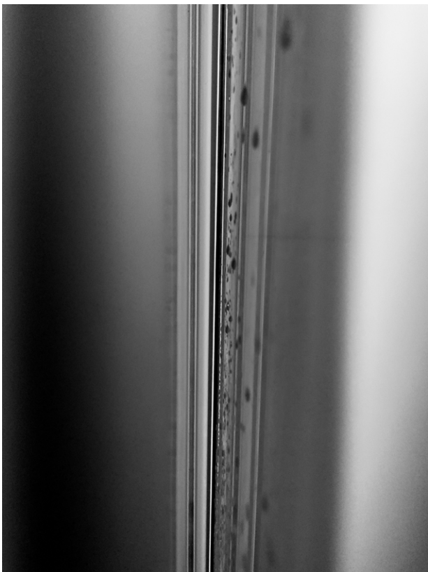
Water stains on acrylic sliding panels
